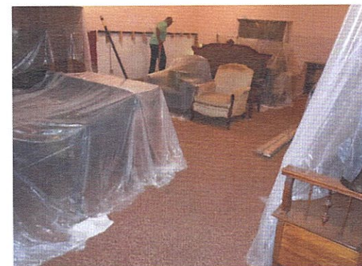
The parlor is in disarray as the waterproofing system is being installed.
