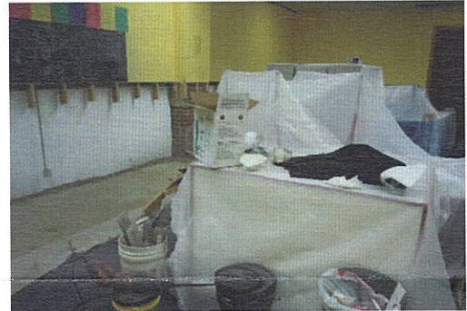
The learning center looks quite different as repairs begin after the water damage.
